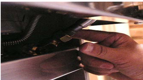
GAS CONNECTION TO GRILL MANIFOLD
